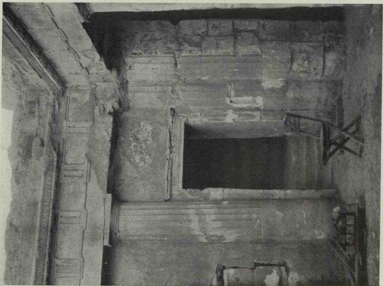
(a) Tombs at Mustapha Pascha, Alexandria. Angle of court showing entry to staircase.
